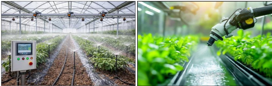
Fig 4 & 5: Automatic Irrigation System inside Greenhouse
